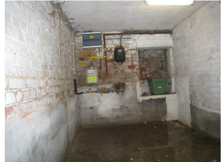
Water in kelder
